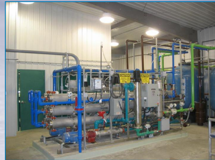
Reverse Osmosis system in operation
